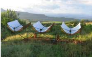
A set of prototype solar concentrators installed in Lesotho. (Courtesy of Amy Mueller.)
